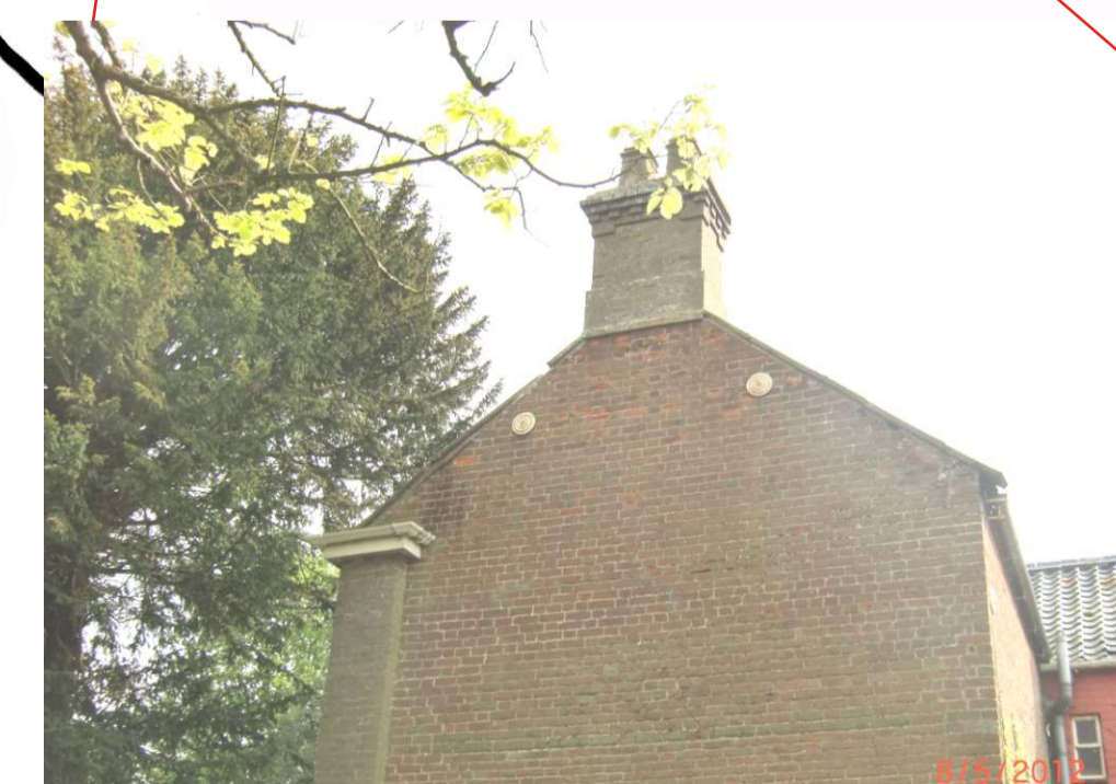
Simple verge detail and front eaves boxing returning around gable (Mill House, Yarmouth Road)
