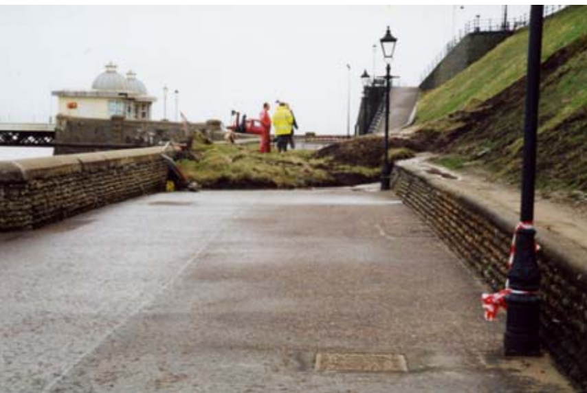
Plates 4.1-4.3 Landslip just west of pier (February 2002)
