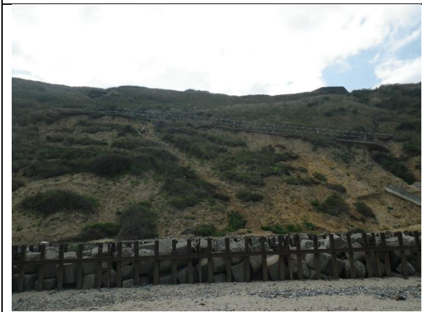
Shallow instability features triggered by toe erosion that are undermining of the lower path.
