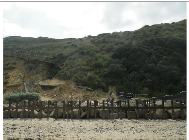
Detail of the lost section fo path caused by toe erosion of Mundesley Sand
