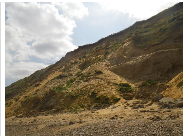
CBU north of the access ramp showing steep cliff and debris falls.
