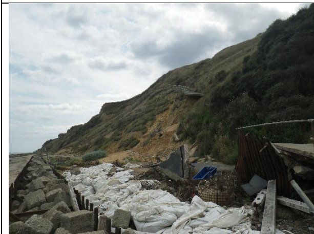
Overview of the lowermost section of path showing undermining of remaining section and toe defences of gravel-filled bags
