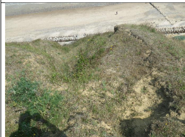
Detail of relict mudslide embayment between the upper and lower sections of path.
