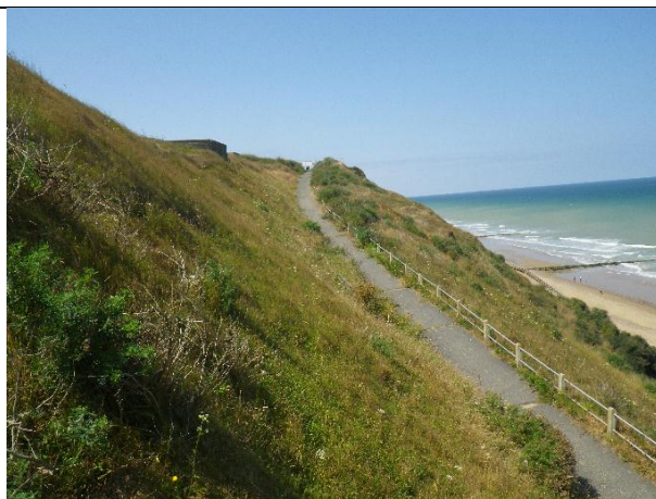
Overview of the upper section of path showing stable slope and footpath in good condition.
