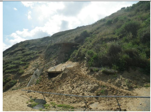
Details of the lowermost section of footpath lost in the December 2013 storm surge. Note the geology here is Mundesley Sand
