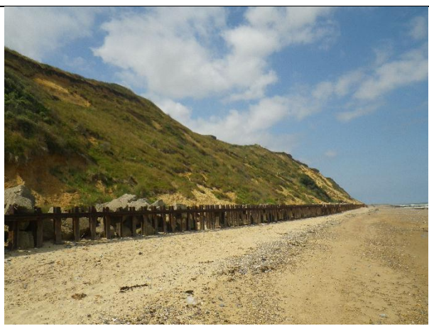
CBU south of the access ramp showing steep slope and localised reactivation of mudslide debris
