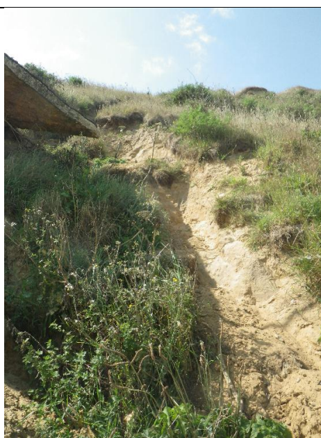
Mudslide embayment that led to loss of the lower-most section of footpath
