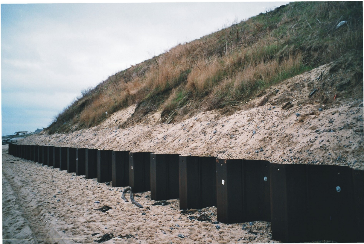
Plate 6 Cliff behavioural unit 19 – view east; note the recent sheet pile wall at the cliff toe
