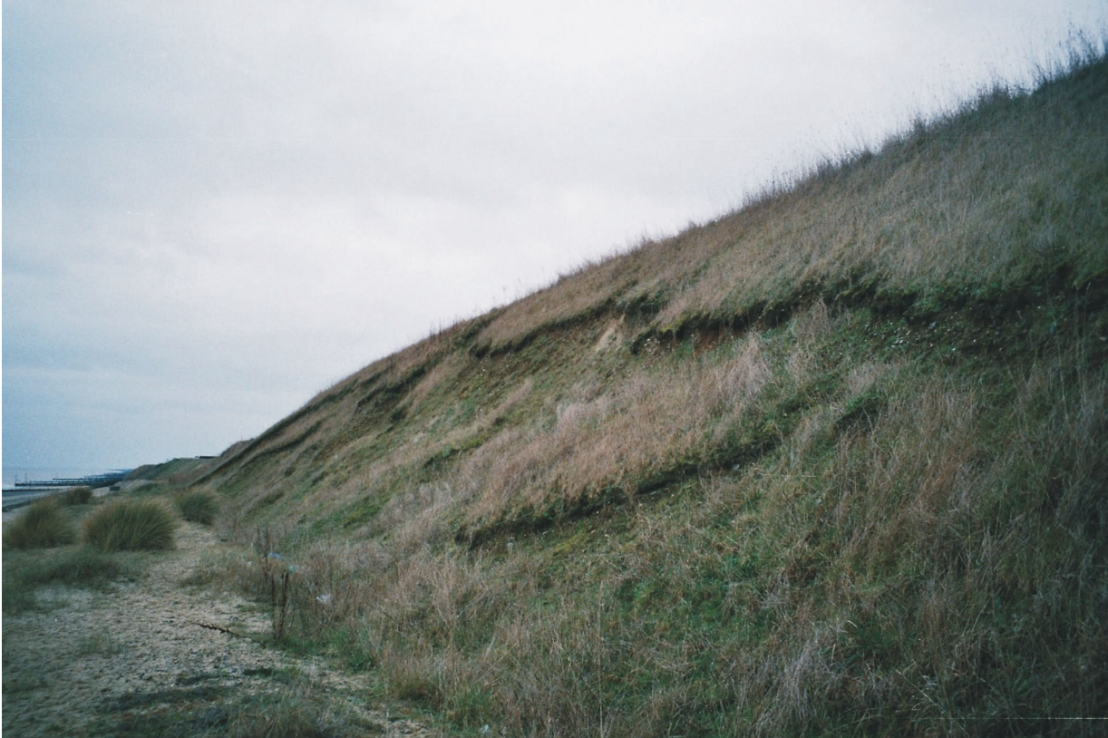
Plate 5 Cliff behavioural unit 18 – view east; note the localised small failures of the regraded slope
