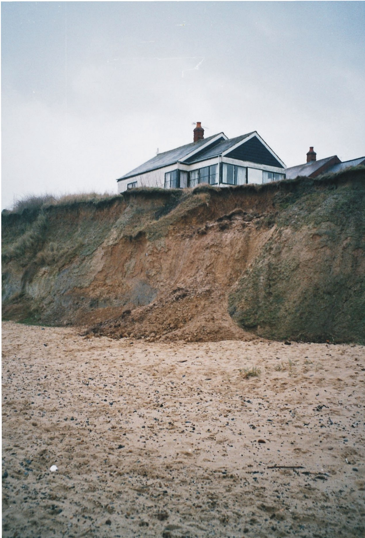
Plate 9 Cliff behavioural unit 21 – Ostend, view east; note the recent small cliff failure
