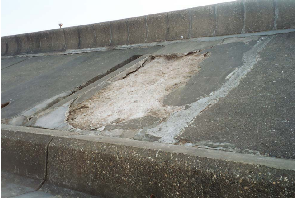
Figure 29 Spalling damage to seawall at Walcott
