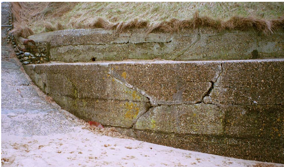
Figure 27 Poor condition of part of old seawall at Mundesley
