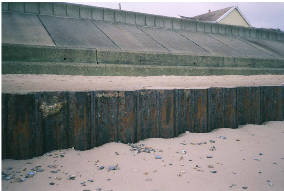
Figure 30 Ostend seawall showing exposed steel sheet toe, low beach level, and washed out jointing
