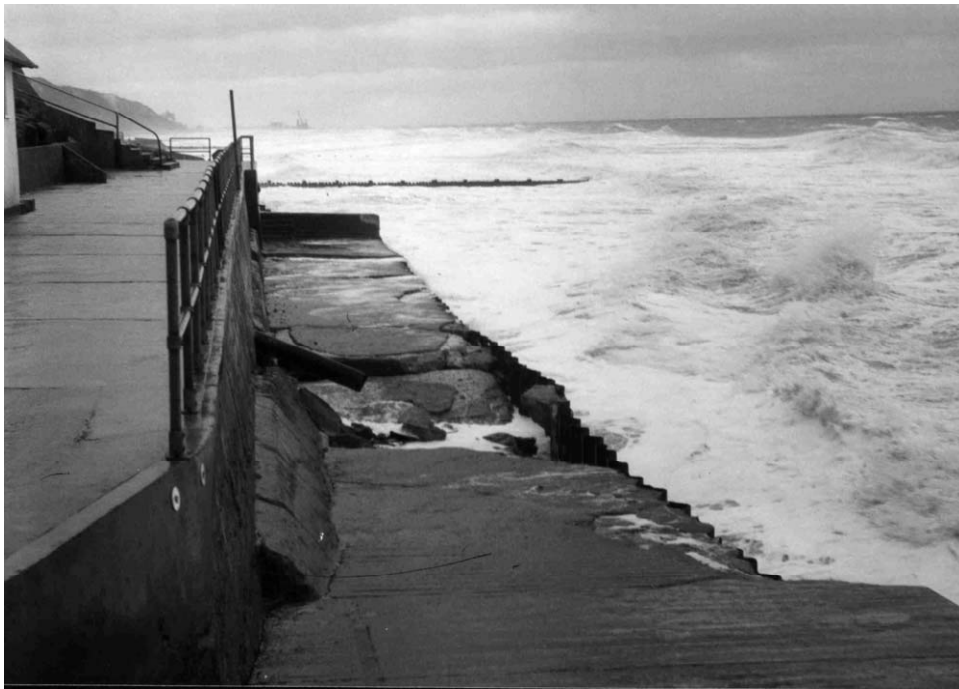
Figure 23 Failure of the apron and steel pile toe in 1997 at Overstrand
