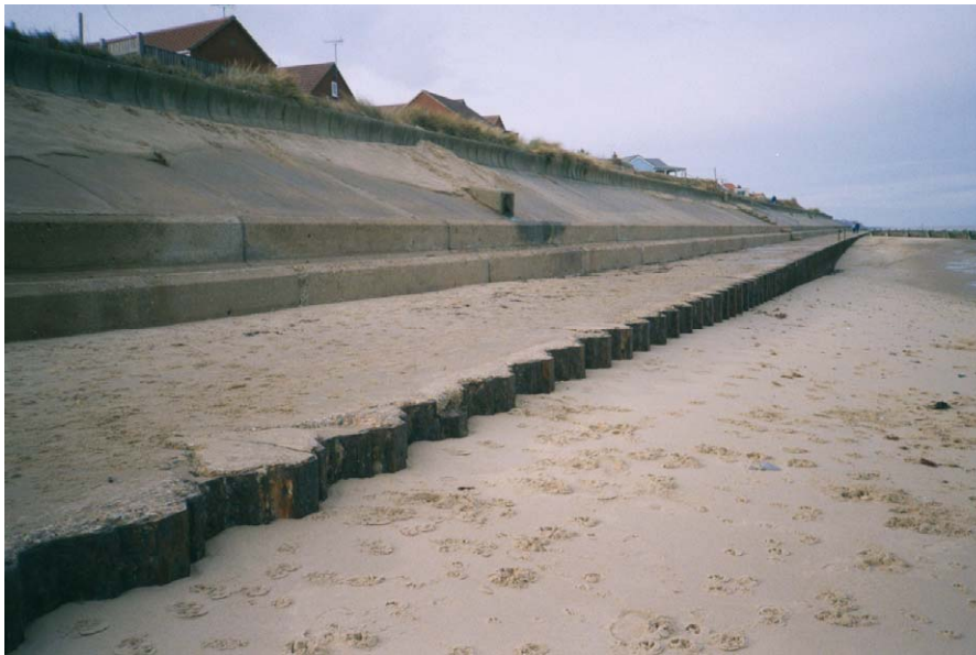
Figure 28 Seawall and steel sheet pile toe at Bacton – note low beach level
