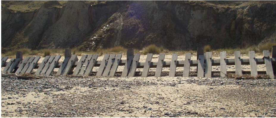
Figure 24 Wooden revetment with boards missing between Overstrand and Trimingham
