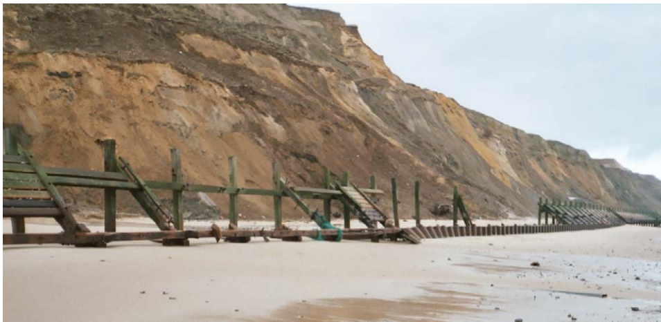
Figure 25 Badly damaged revetment and piles
