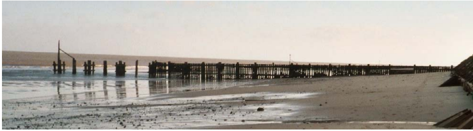
Figure 26 Failure of seaward end of a groyne
