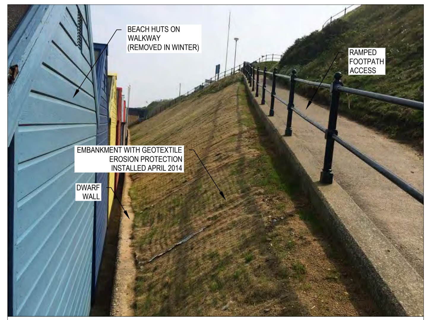
PHOTOGRAPH OF EXISTING EMBANKMENT (NOTE EXISTING GEOTEXTILE EROSION PROTECTION REPAIR UNDERTAKEN IN 2014)
