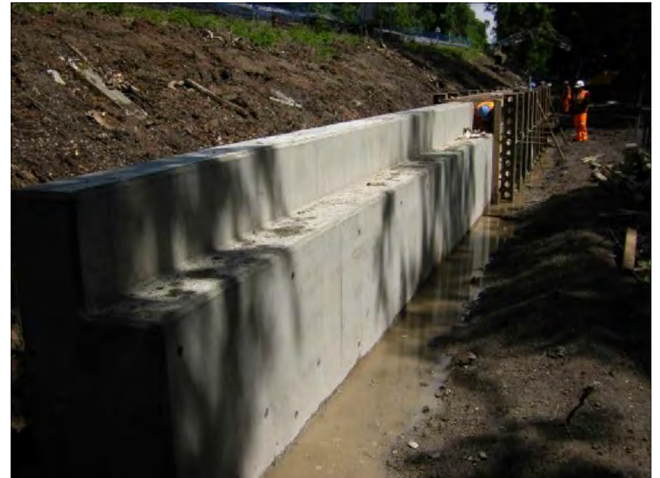
EXAMPLE OF UPSTAND WALL SCOUR PROTECTION PHOTOGRAPH COURTESY OF TAG CONSTRUCTION LTD
