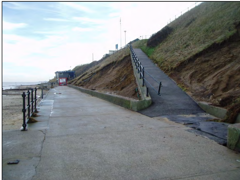
Figure 1-2: Photograph of embankment scour failure following December 2013 storm event (courtesy of NNDC)
