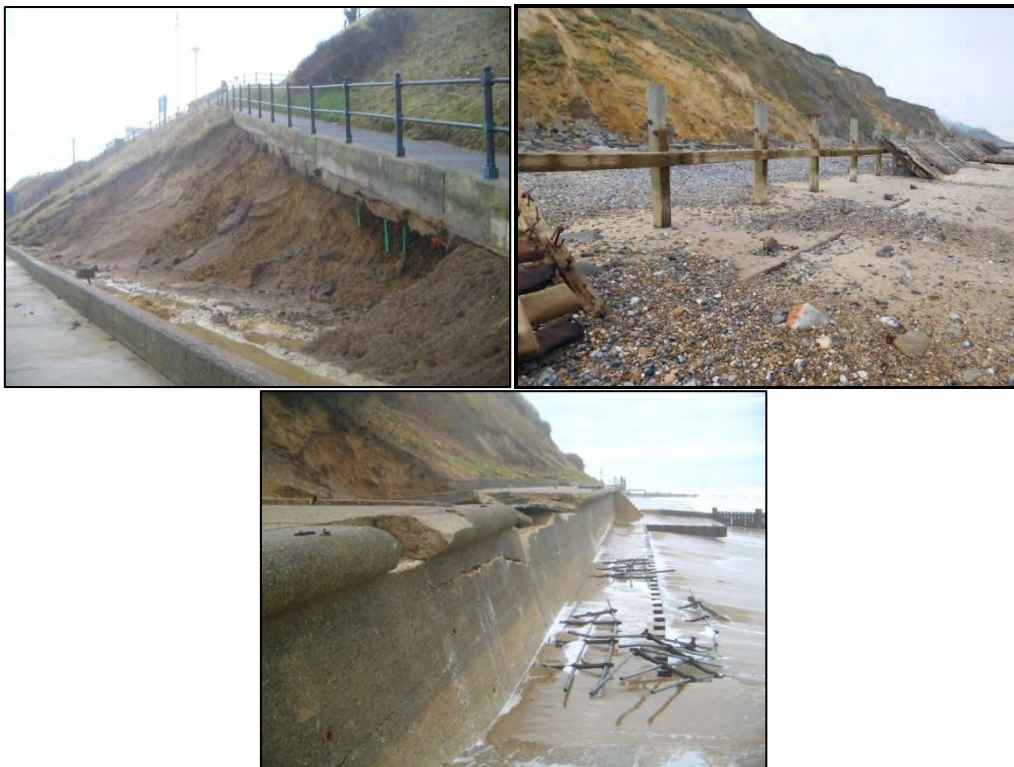
Figure 2.1 – Typical Winter Storm Damage
