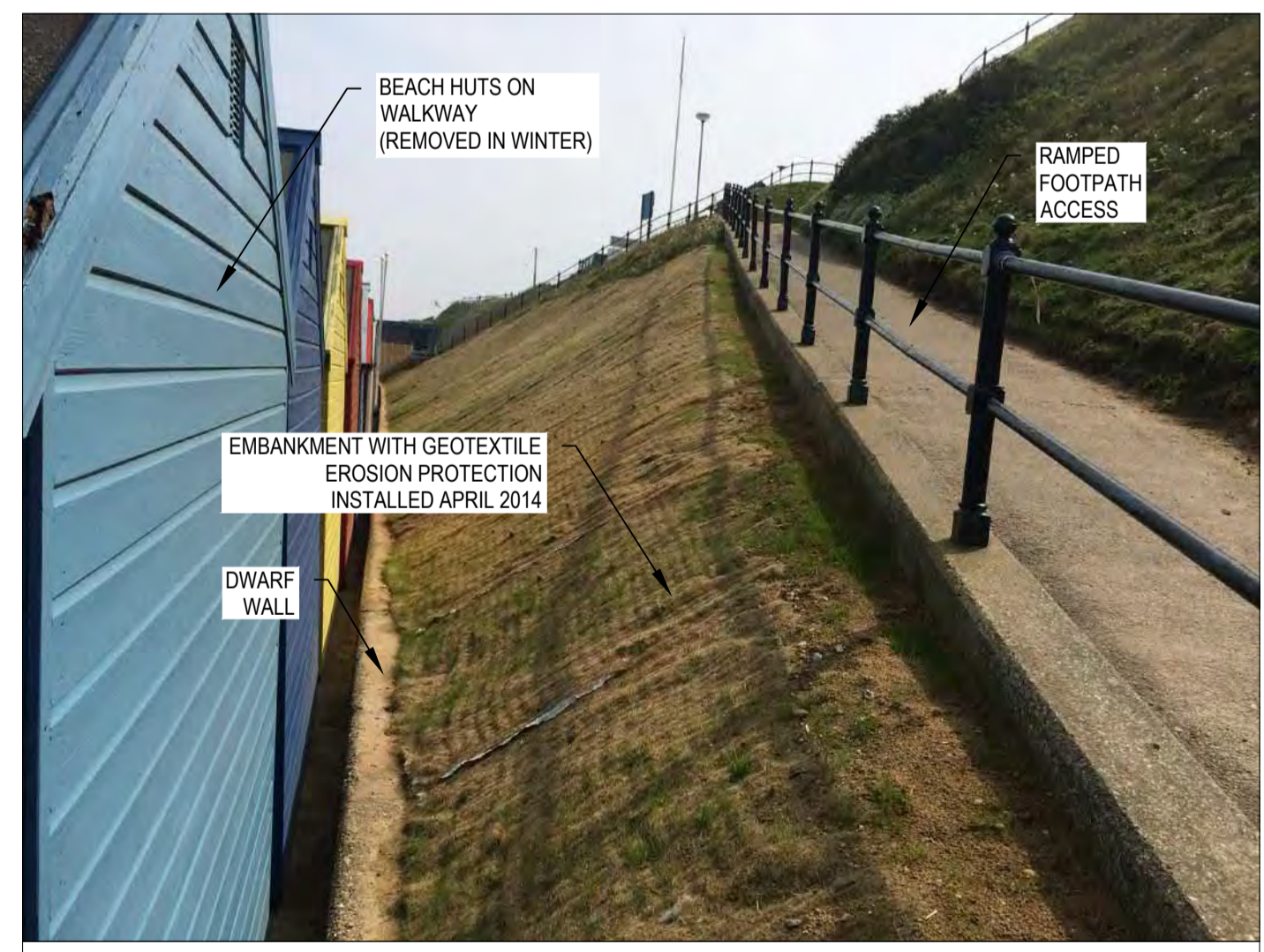
PHOTOGRAPH OF EXISTING EMBANKMENT (NOTE EXISTING GEOTEXTILE EROSION PROTECTION UNDERTAKEN IN 2014) PHOTOGRAPH COURTESY OF NNDC, APRIL 2014
