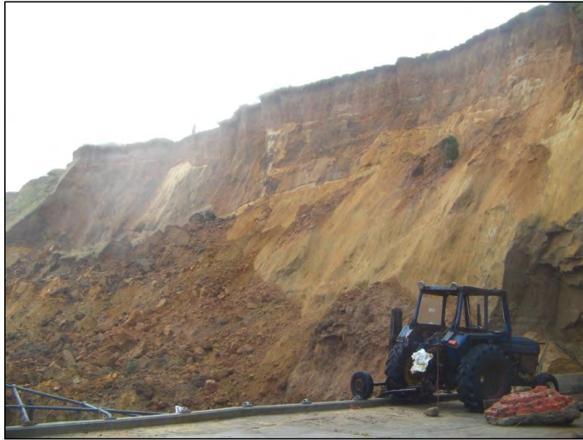
Figure 1-1: Photograph of cliff failure (erosion) following December 2013 storm event (courtesy of NNDC)
