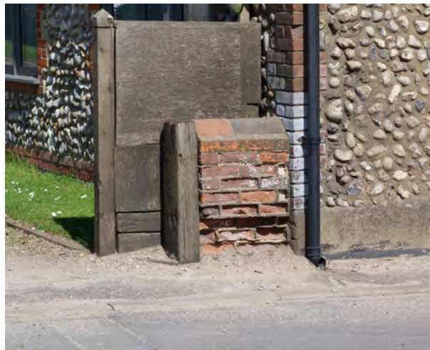
Worn bricks, caused by water splashing up from the road from passing vehicles
