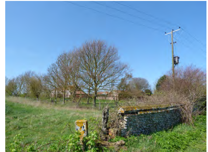
Damaged wall at south-east corner of the Conservation Area [NB: not currently in Conservation Area but would be if boundary was amended]
