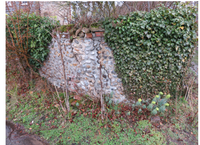
Damaged flint wall along The Street
