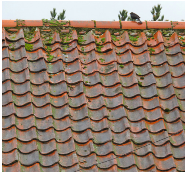
Moss on a roof affects the appearance of the building but also holds moisture against the tiles. The moss also blocks gutters and drains when it is dislodged
