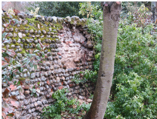
Failing flint wall on Chapel Lane
