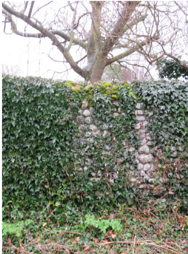
Ivy engulfed wall on Chapel Lane
