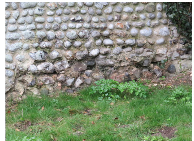
Failing flint wall on Leatherpool Lane
