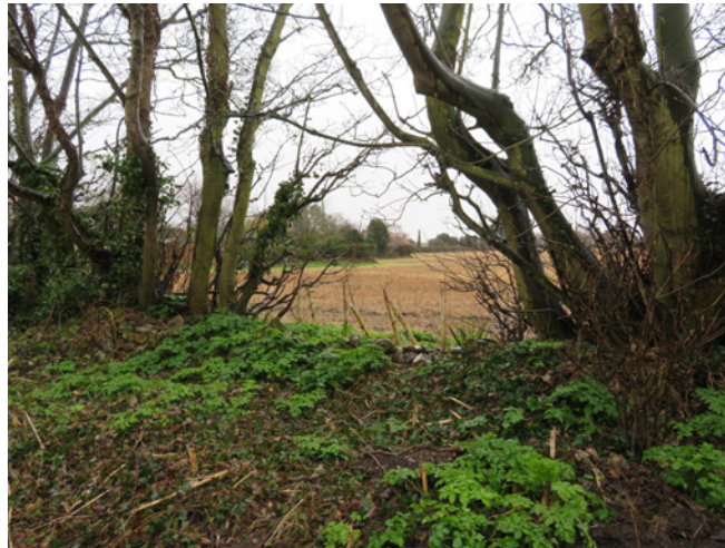
Collapsed flint wall along The Street
