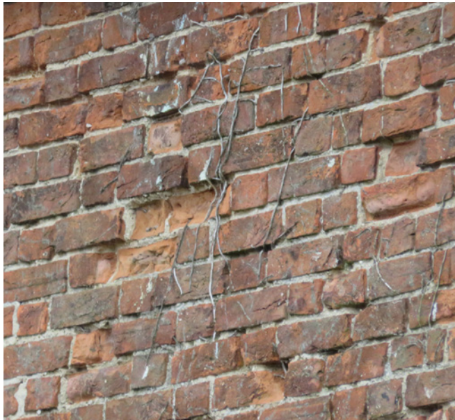
Norfolk bricks are typically soft and prone to erosion especially if the pointing is not maintained
