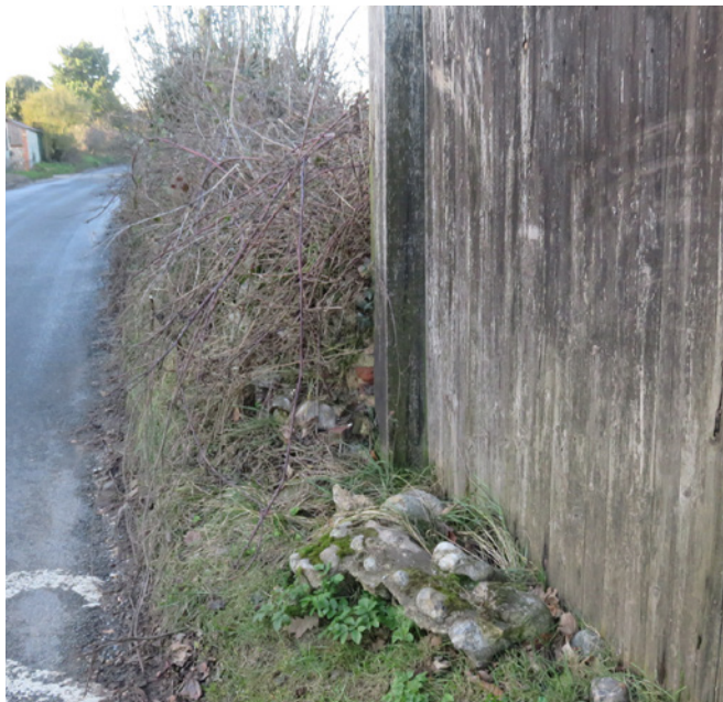
Engulfed and failing flint wall on Blakeney Road
