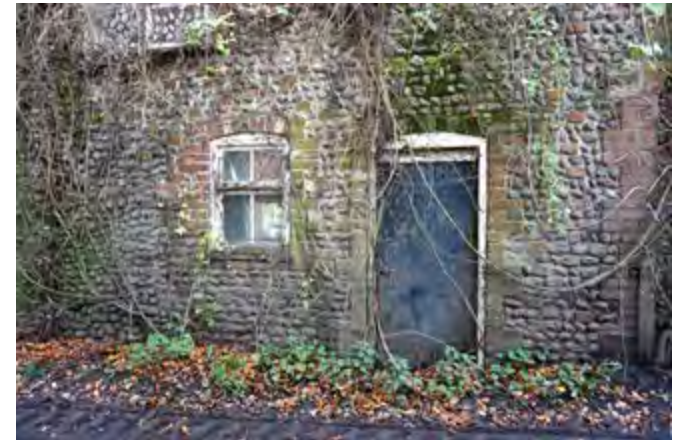
Timber work in poor condition
