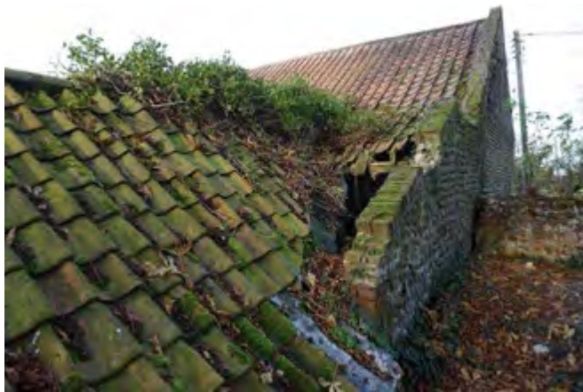
Barns in poor condition as seen from the churchyard
