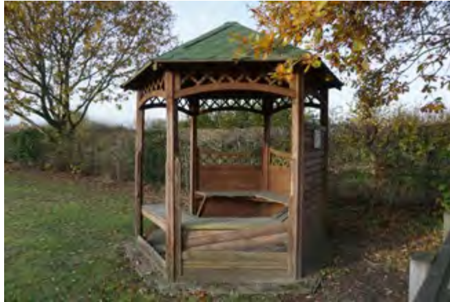
Damaged shelter at the playground
