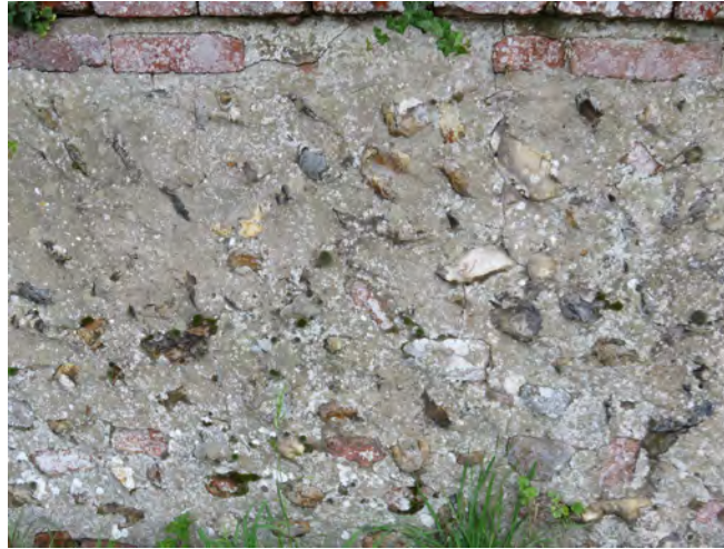
Excessive repointing to flint wall
