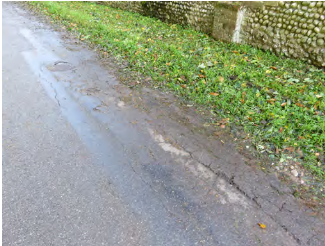
Poor road surface on The Street
