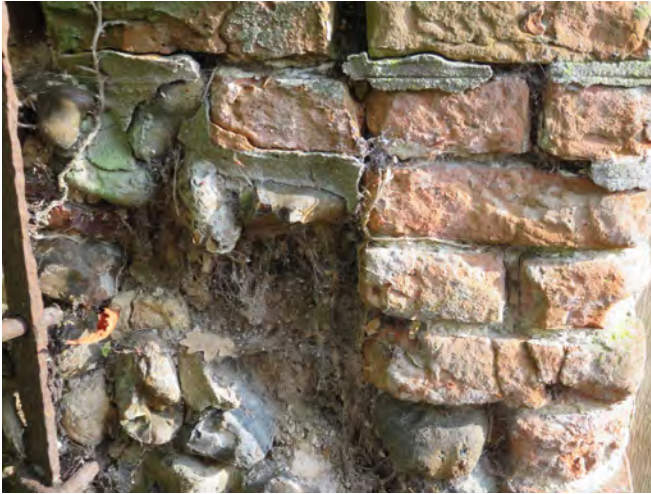
Cementitious repointing, missing flints and damaged bricks to a historic boundary wall
