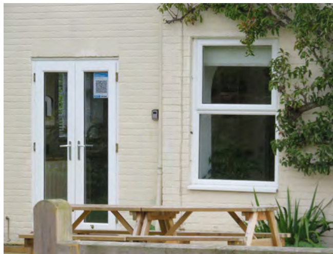
Inappropriate uPVC door and window
