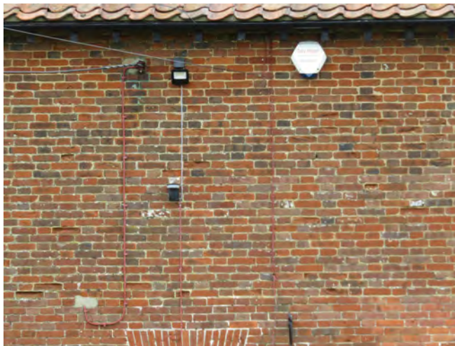
Accumulation of cables, light and security alarm
