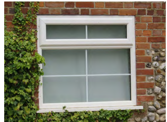
Inappropriate uPVC window
