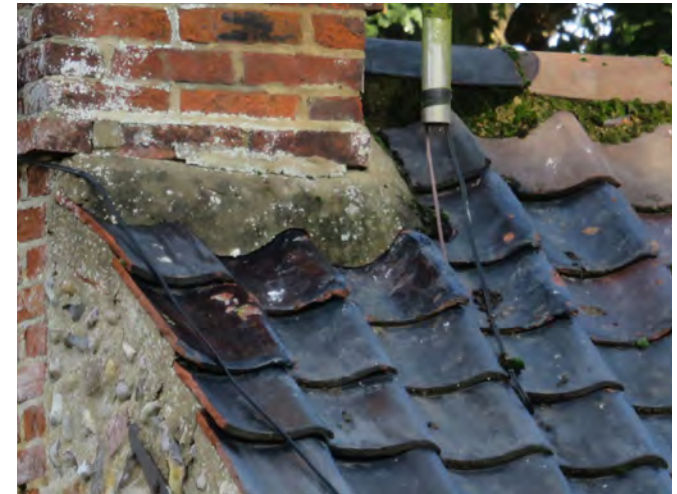
Inappropriate cementitious repairs to chimney and roof
