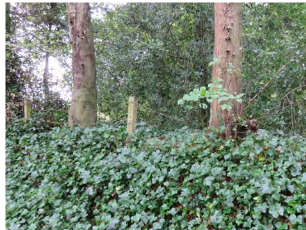
Poor quality post and barbed wire fence in poor condition
