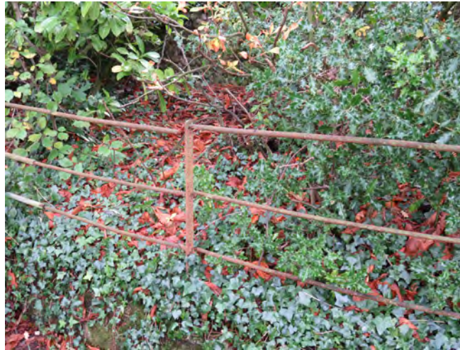
Broken and corroding railings
