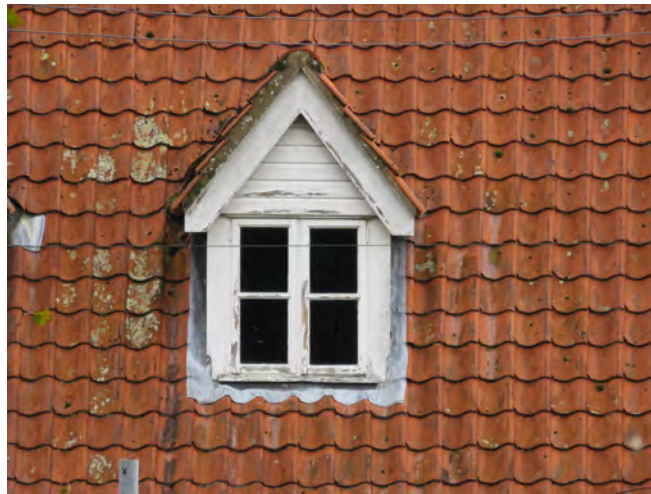
Window joinery that requires repainting
