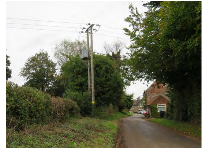
Pylon on The Street
