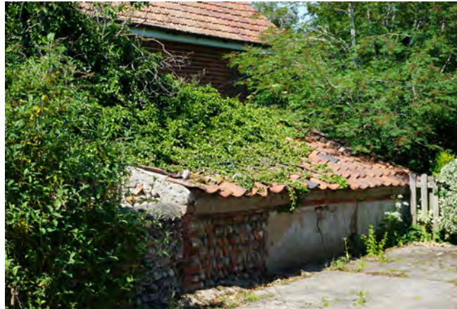
Outbuilding in poor condition with overgrown vegetation
