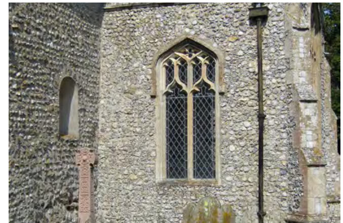
Detail from south elevation of the church showing two phases of windows
