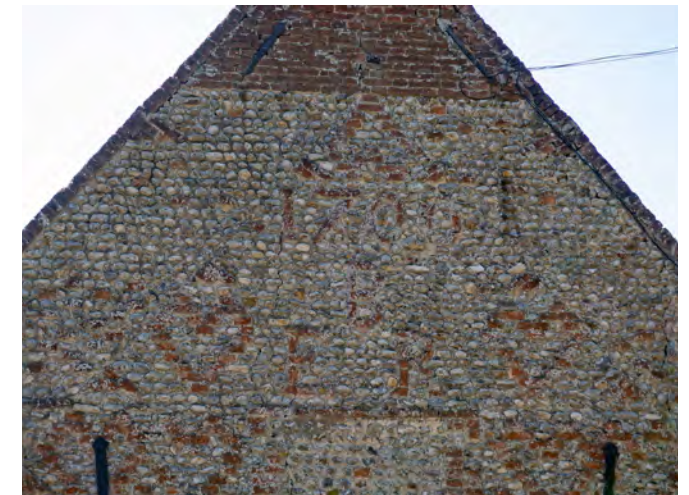
Brickwork patterns in the south gable of the large barn at Hunworth Hall, reading '1700 B E R'
