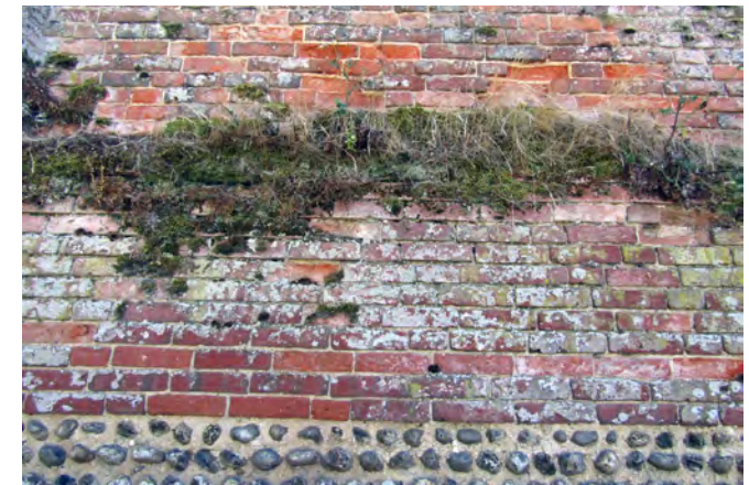
Vegetation growth to a wall
