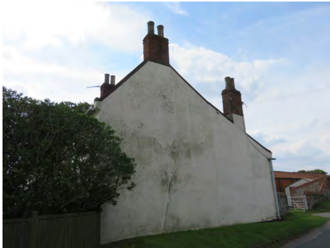
Damp issues seen on external render
