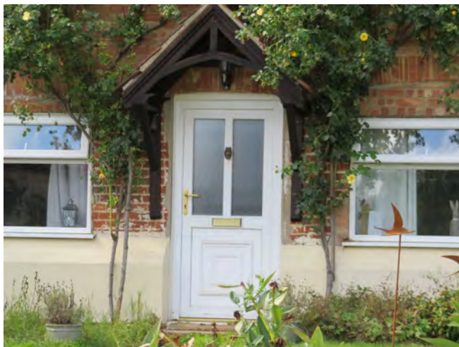
uPVC door and windows
