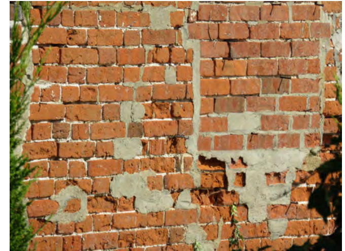
Eroded historic bricks due to cementitious pointing
