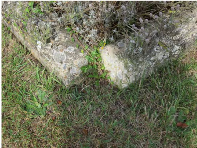
Three cornerstones are missing from the war memorial
