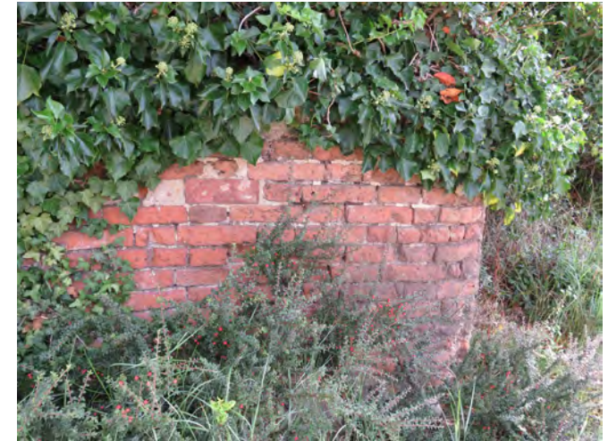
Vegetation growth on brick wall
