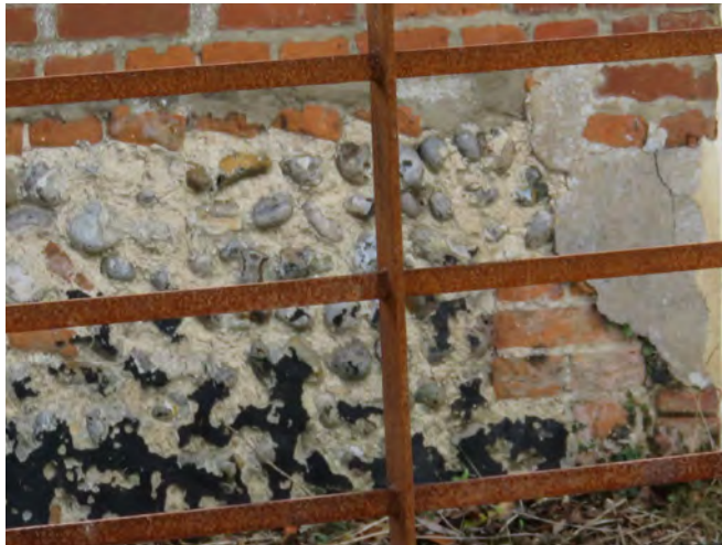
Inappropriate concrete repair
