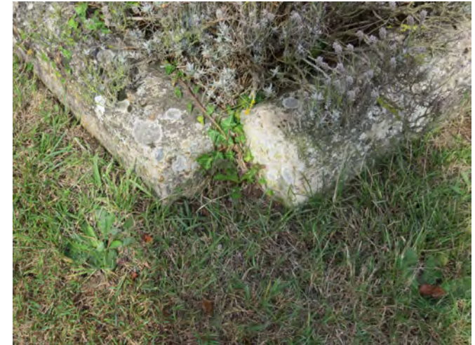
Cracked concrete base of memorial with vegetation growth
