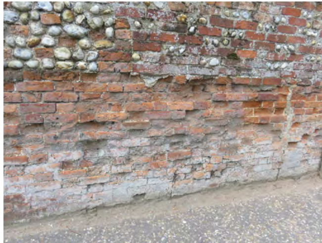
Erosion of brickwork caused by spray from the road
