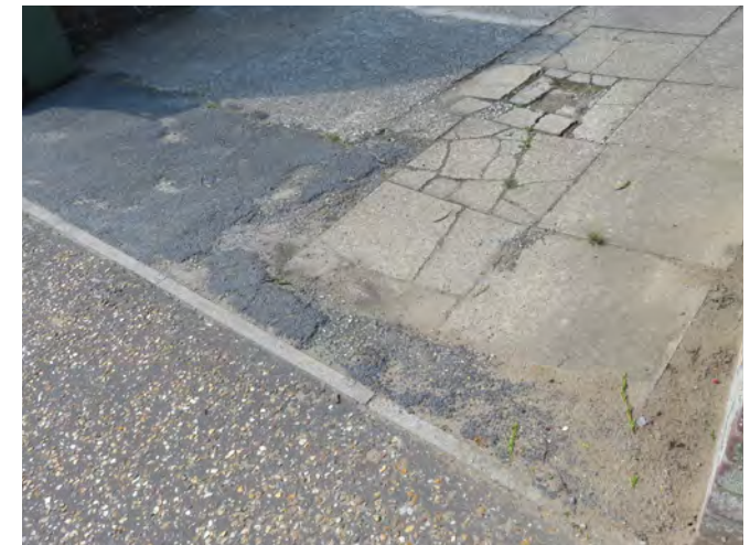
Cracked paving slabs on driveways
