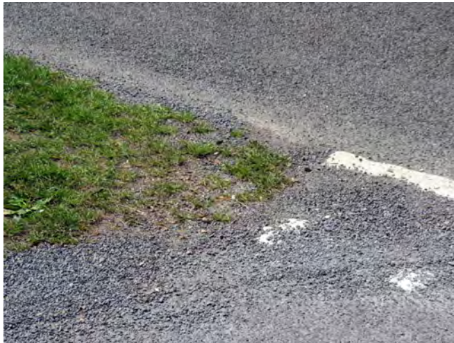
Worn corners to the junctions are common in the village
