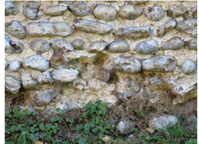
Eroded pointing causes loss of flints
