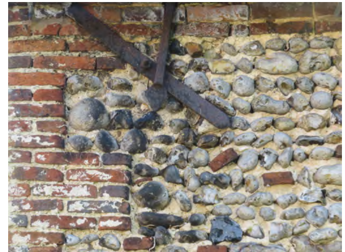
Regular overspilling of water from missing, damaged or inadequately sized rainwater goods causes damage to the historic fabric
