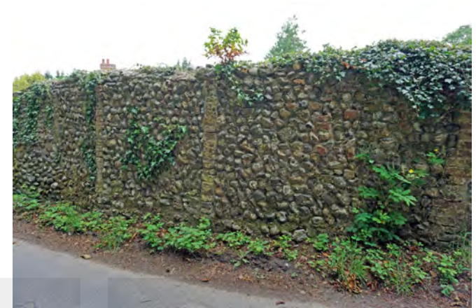
Section of red brick and flint wall fronting the graveyard of Stody Church shown with patches of vegetation growth
