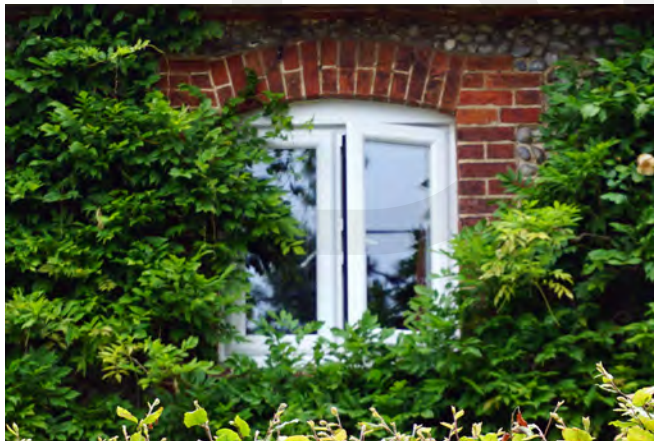
Inappropriate uPVC windows
