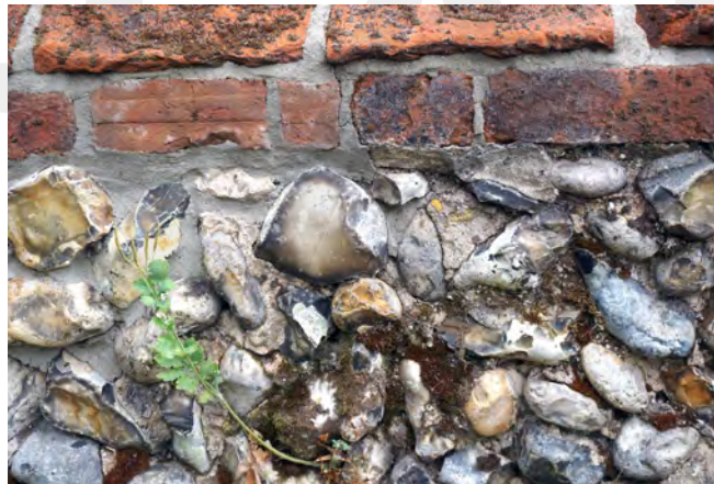
Cement pointing to an historic wall
