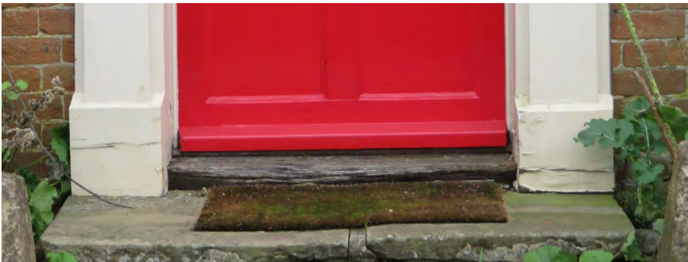
Rotting base to doorcase
