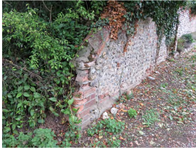
Damage to a wall compounded by cementitious pointing
