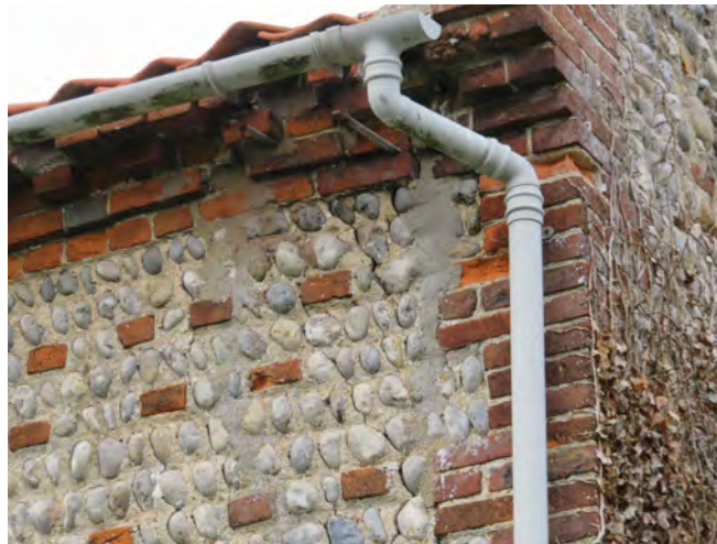
Cracks and cementitious repairs to a building
