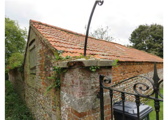
Damage to the capping of the gate pier to the churchyard
