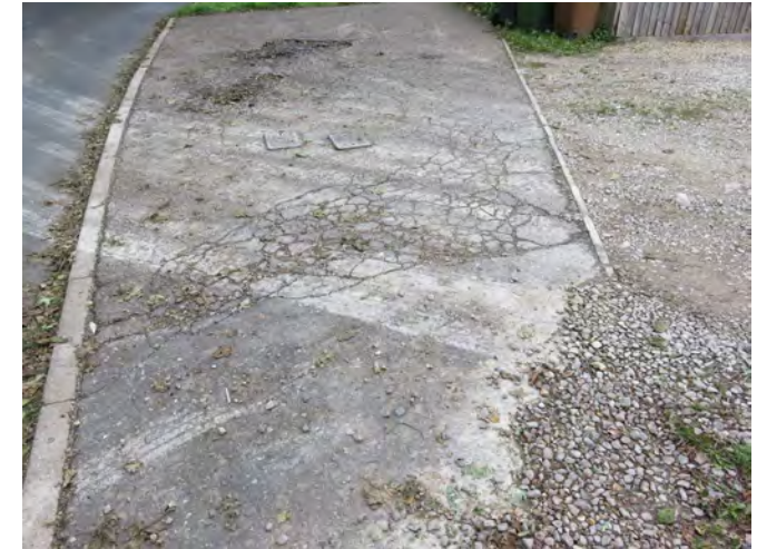
Poor surfacing to a large access splay
