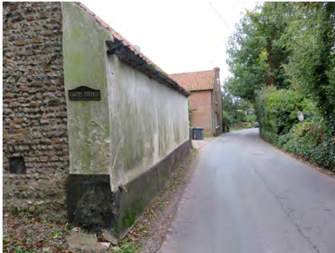
Missing drainpipe and evidence of building being struck by a vehicle on the main road
