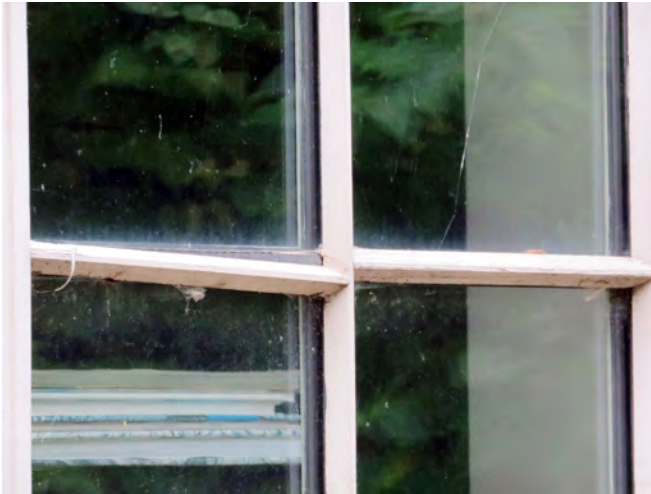
Glazing bar that has come unstuck on a slimline double glazed replacement window
