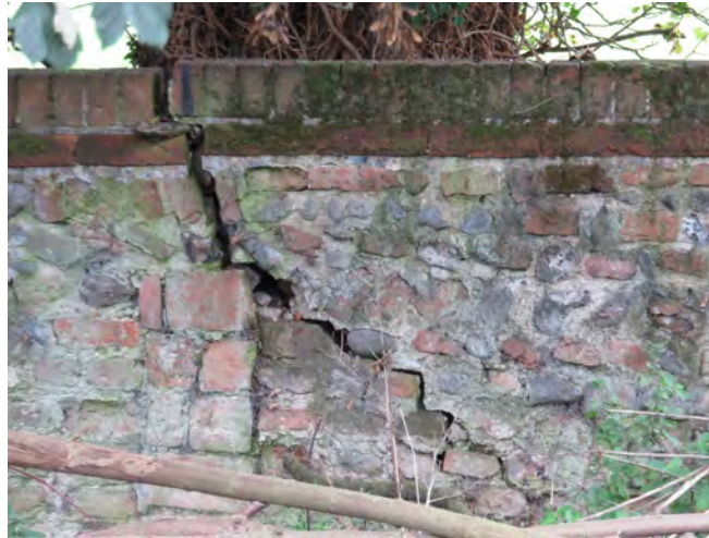
Cracked boundary wall due to tree growth
