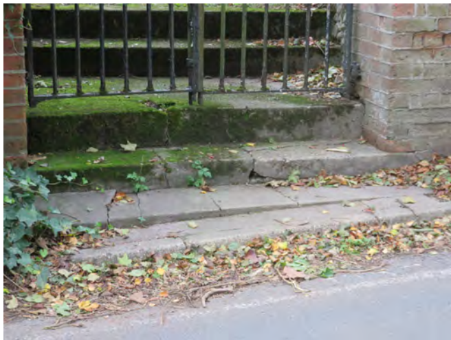
Cracking cementitious screed to steps
