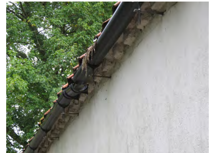
Broken gutters cause water to soak the walls, which leads to deterioration of the fabric
