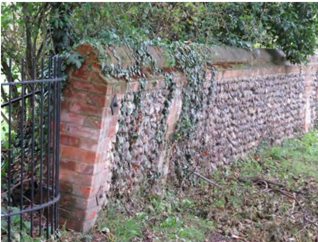
Leaning boundary wall
