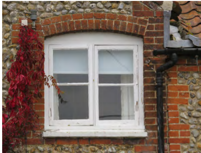
Example of external timber joinery requiring repainting
