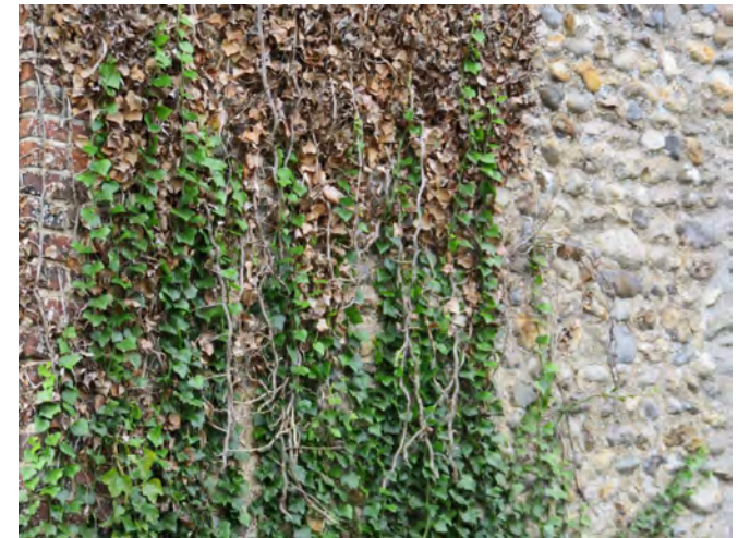
Ivy growth causes damages to historic fabric, as can its removal if not undertaken carefully
