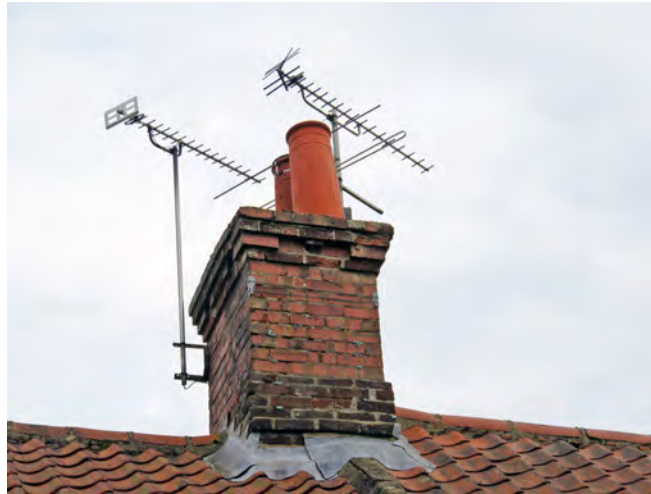
Television aerials and associated supports and cabling detract from the appearance of historic buildings and can cause damage to the historic fabric.
