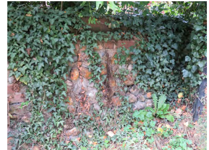
Vegetation growth causing damage to the brick and flint boundary wall
