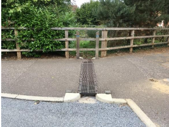
Photo of a rill from a carriageway through a path to a SuDS Basin – Drayton, Norfolk (image E Simpson @ NCC LLFA)
