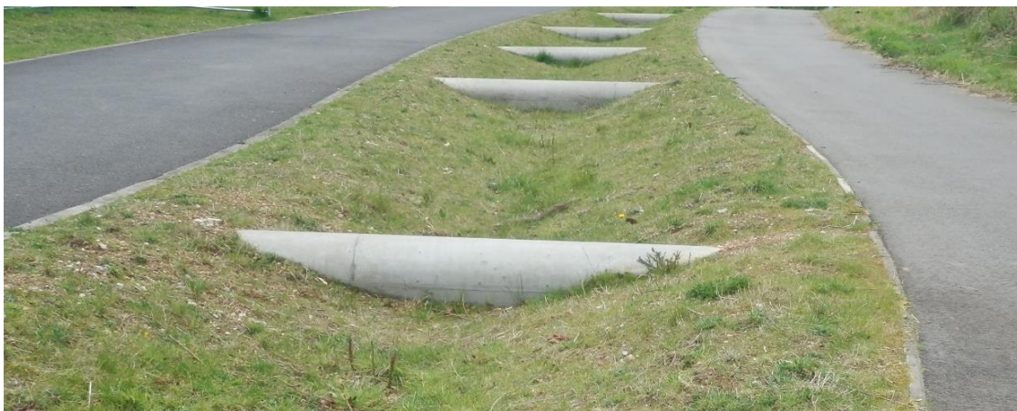
Photo of a swale draining the highway (bus lane and shared use path) located at Queens Hill development, Costessey, Norfolk (image E Simpson @ NCC LLFA)
