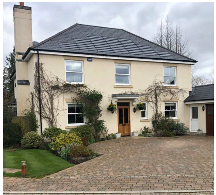
Figure 87: Use of shingle-like solar panels on a slate roof, with the design and colour of the solar panels matching those of the adjacent slate tiles in Lingfield, Surrey.
