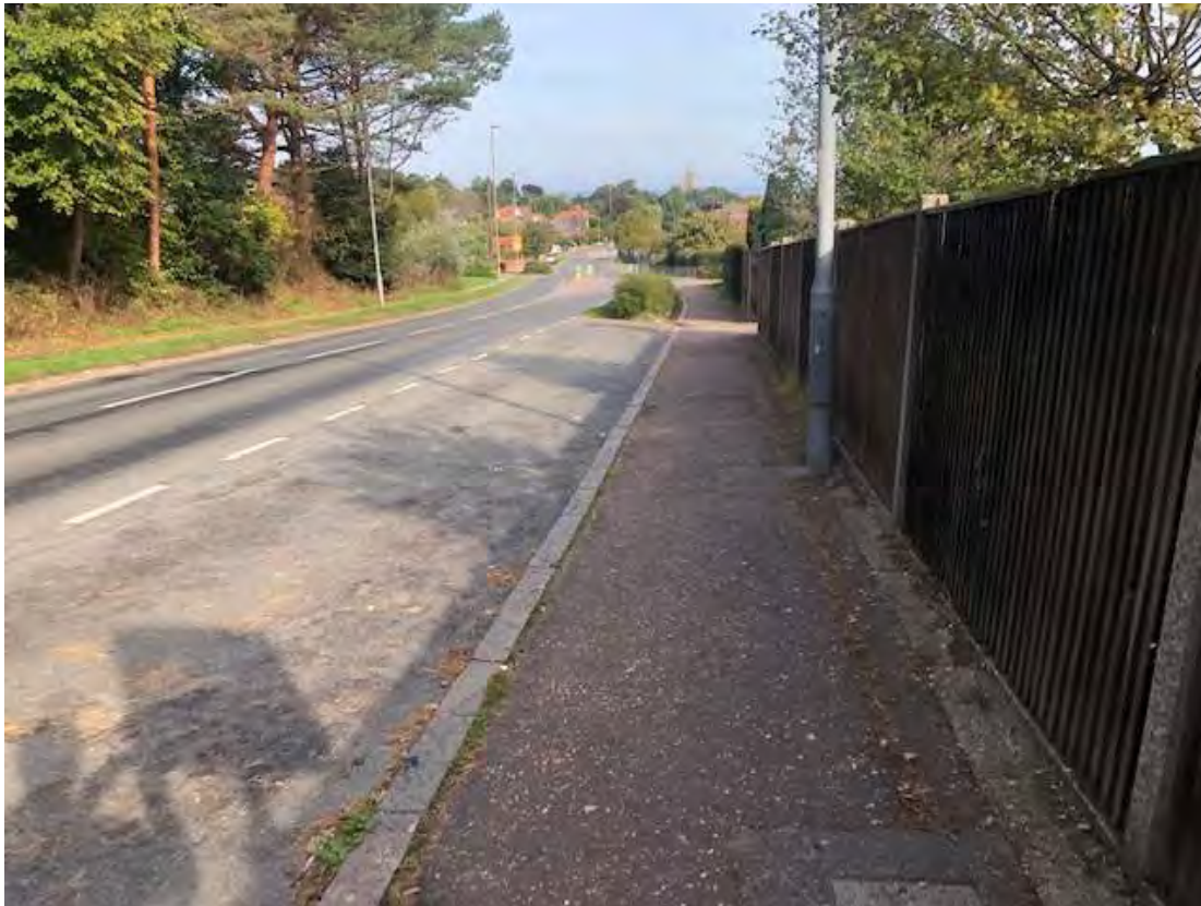
FIG 28 EASTERN FOOTWAY OF NORWICH ROAD LOOKING TOWARDS CROMER ACADEMY- NO TACTILE PAVING
