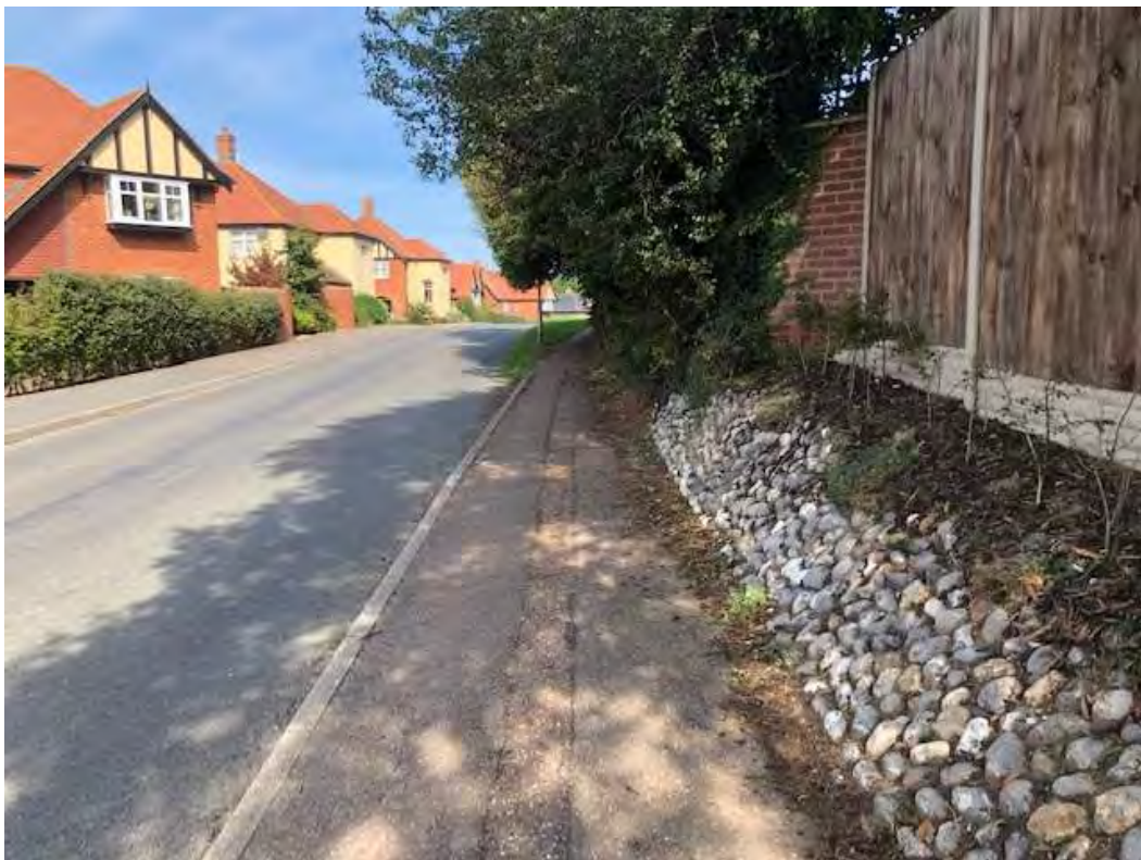
FIG 63 EASTERN FOOTWAY ROUGHTON ROAD NORTHWARDS- BUSHES NEED CUTTING BACK
