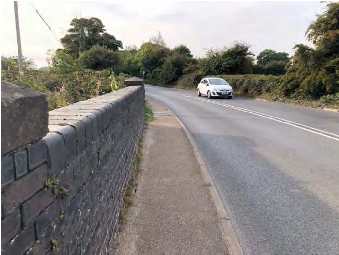
FIG 5 VIEW SOUTHWARDS ON OVERBRIDGE EASTERN FOOTWAY -RESTRICTED WIDTH
