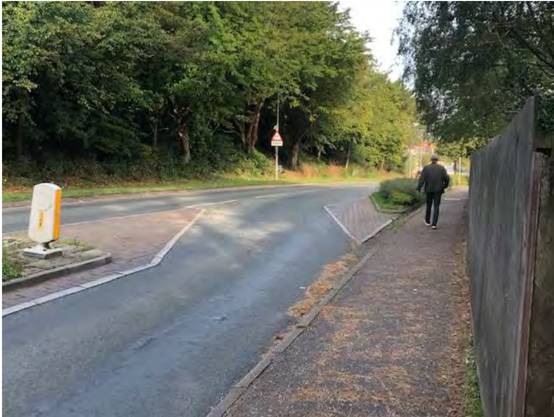
FIG 26 EASTERN FOOTWAY OF NORWICH ROAD ADJACENT TO TRAFFIC CALMING WHICH DIRECTS TRAFFIC TOWARDS FOOTWAY
